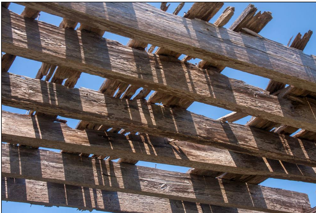
Figure 27. Stringers and deck of North Channel Bridge from Pamlico Sound (photographer: Michael Henderson, January 30, 2016)
