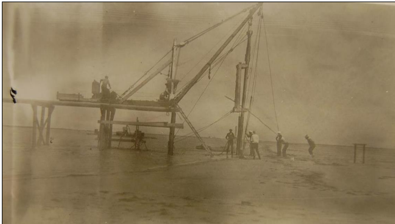
Figure 5. North Channel Bridge: caption reads “Pile Driver at Work”; note top-down method of construction (State Highway Commission, n.d.)
