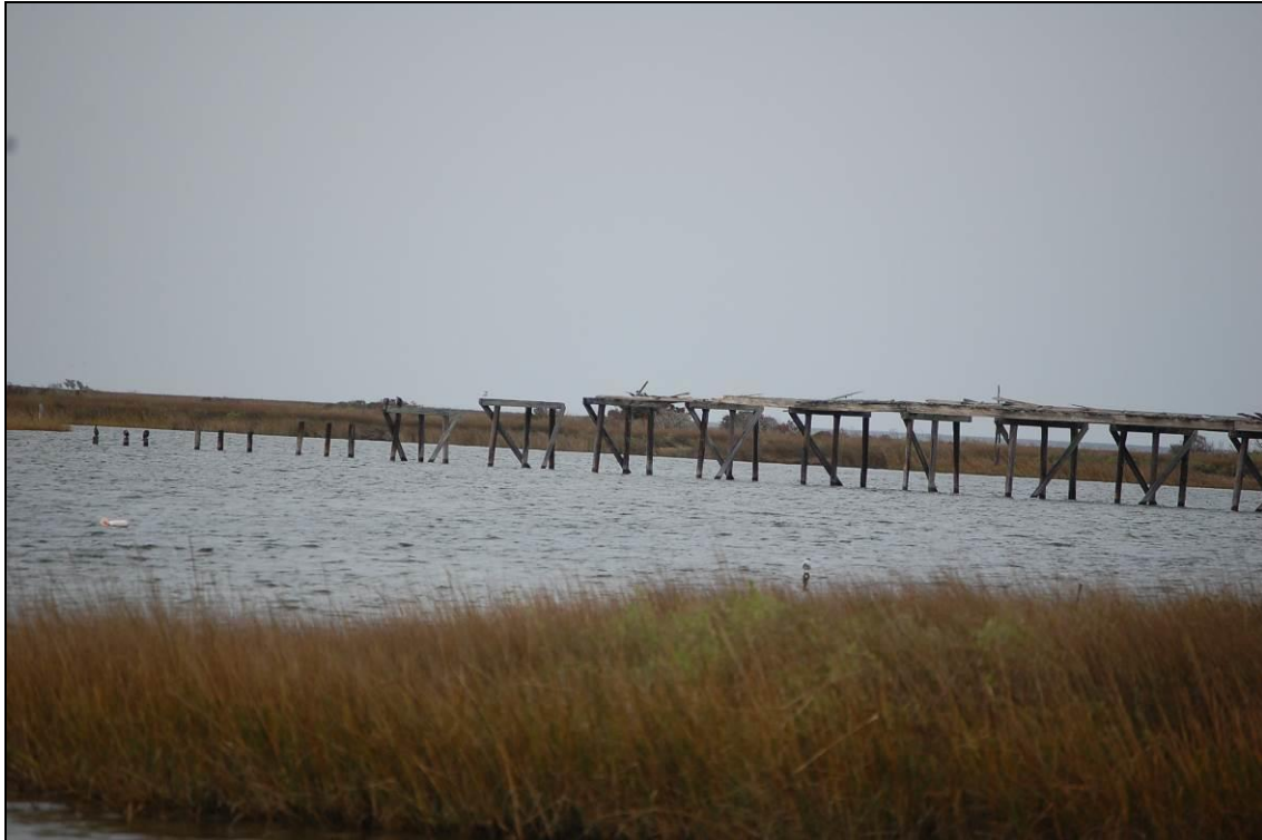
Figure 28. Southern end of North Channel Bridge from NC 12 (photographer: Marvin Brown, November 9, 2016)
